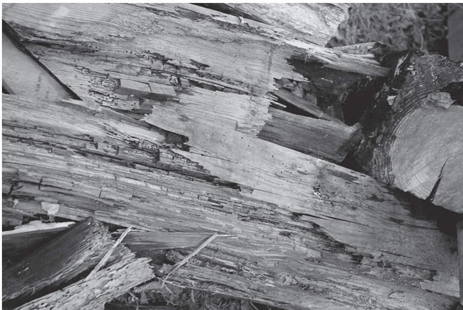
Fig. 1. Fragment of the destroyed roof framing construction
